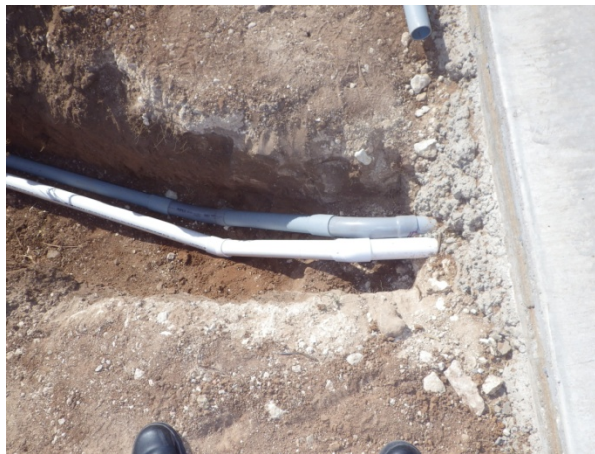
(Above) Conduit from Slab to Control Room with compound shape fitted and glued by students.
