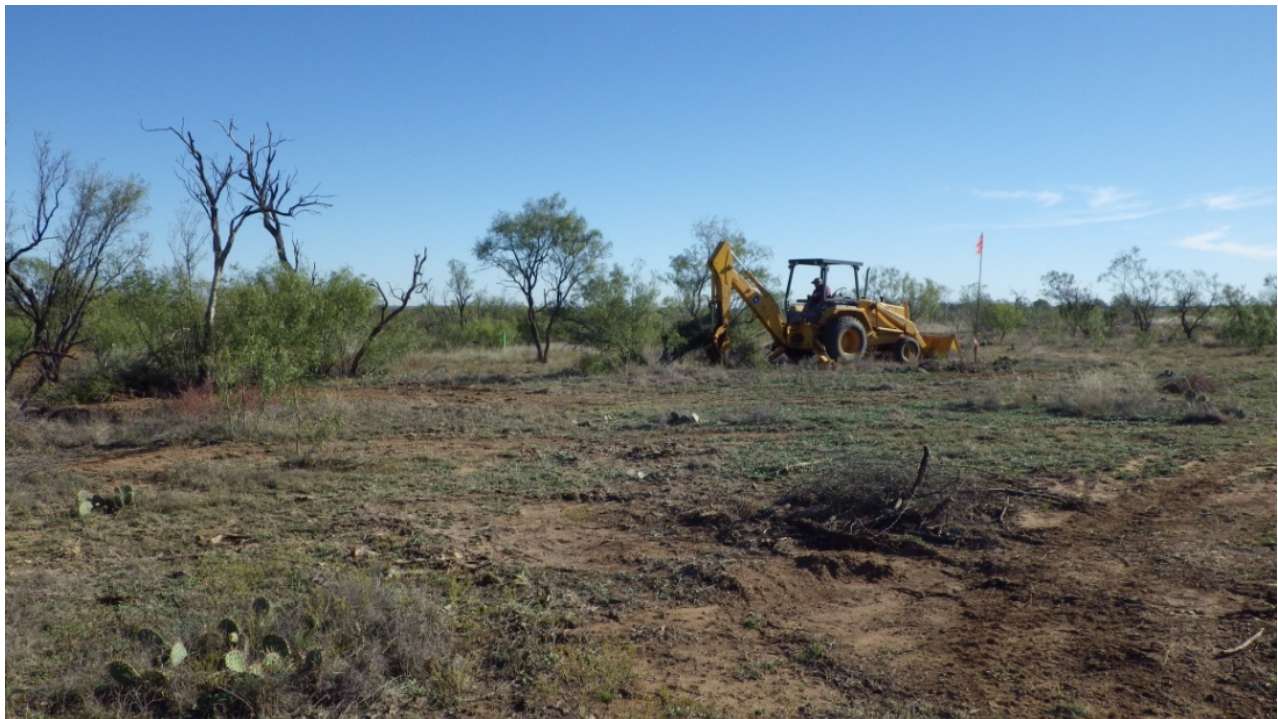
(Above) Prior to installation of the power line, a “Right of Way” had to be cleared through the interior portion of the field lab.
